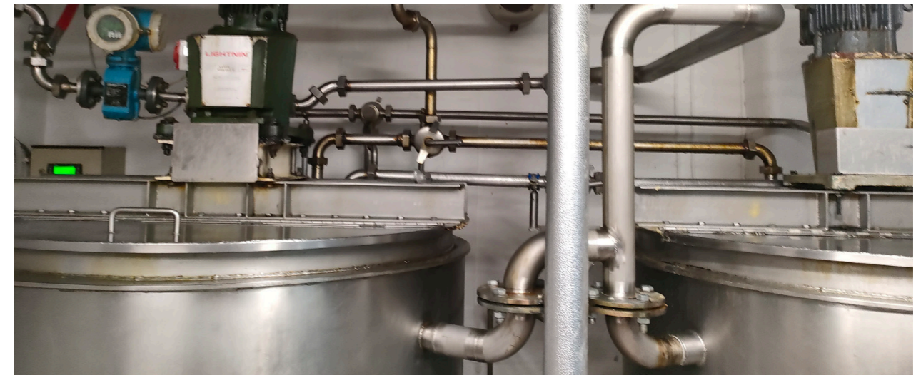
Figure 2: New tanks in position with new lids and new pipework connected to old
